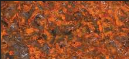
Without corrosion protection treatment
